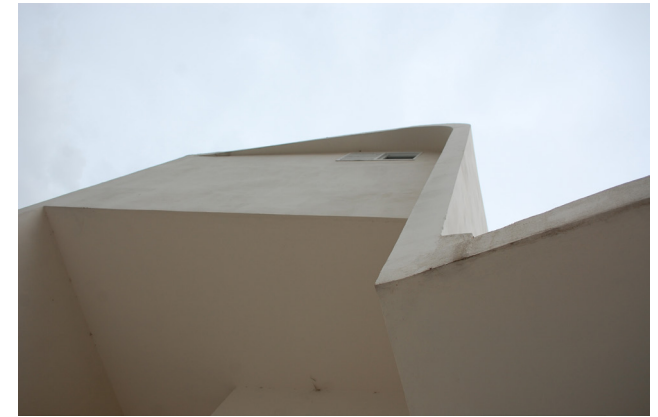
Detail of the Main Elevator Machine Room Modelle Ocampo Building, Buenos Aires, Argentina
